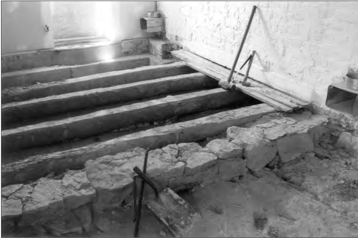
Figure 5. View from room block #4, of the log and plank floor being removed from room block #3. In the foreground is the interior dividing wall foundation, to the right is the central wall of the house. Upper left is the gable end wall that has been stabilized with a new concrete foundation.
