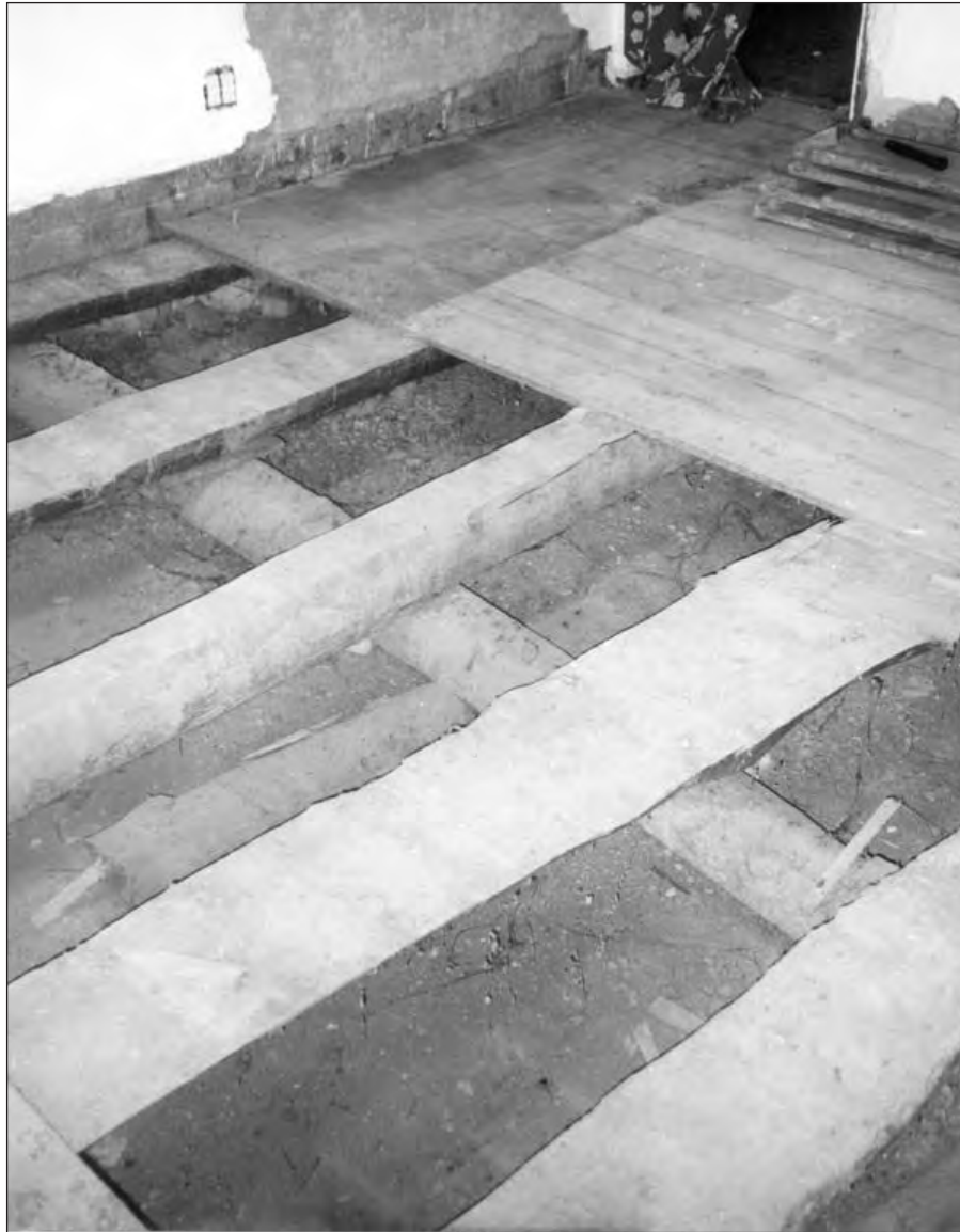
Figure 11. Photo of the central support beam floor in room block #2. The doorway leading to room block #4 is at the upper right.
